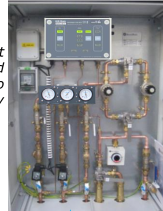
View inside panel
