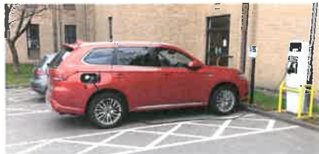
Vehicle connected to the electric charging point at Dewsbury hospital
