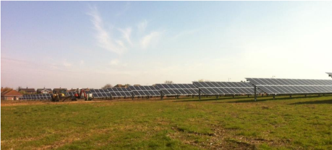
Figure 15 Photovoltaic installation at the James Paget NHSFT
